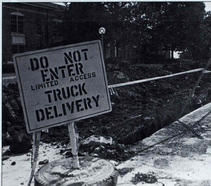
Excavation work leaves the parking lot west of Science Hall as a no-parking zone. Not only were students and faculty forced to park farther away from the building's entrance, but they were also unable to enter through the western doors. (photo by Dave Mullison)
