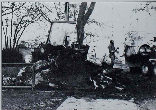
The future home of Northeast's clocktower adorns the campus near the Student Union Building. The scaffolding and plastic sheets were all students saw during the building phase. The clocktower was one of the final expansion phases to $14 million Pickler Memorial Library. (photo by Dave Mullison)
