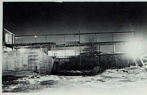
The beginnings of the Natatorium which is scheduled for completion early in 1976.
