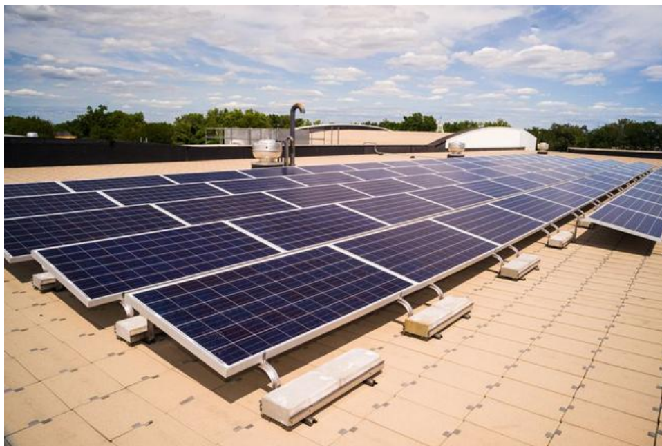
Solar panels were added to five buildings on the University campus to reduce energy consumption and increase sustainability.
